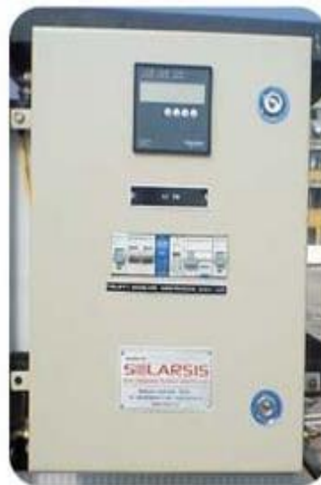
AC Metering Box
