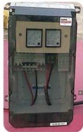
DC Junction Box
