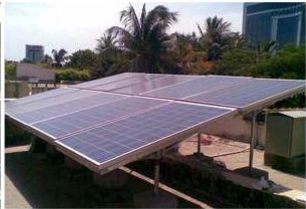
3KW Rooftop Solar PV System
