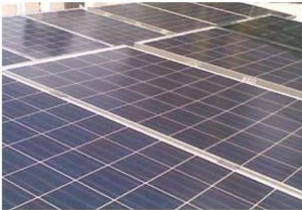
2.25KW Rooftop Solar PV System
