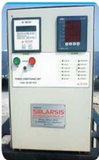
Power Conditioning Unit
