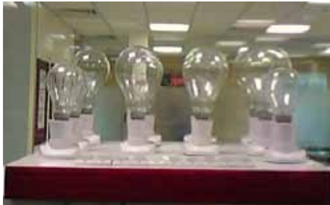
Resistive Load Bank
